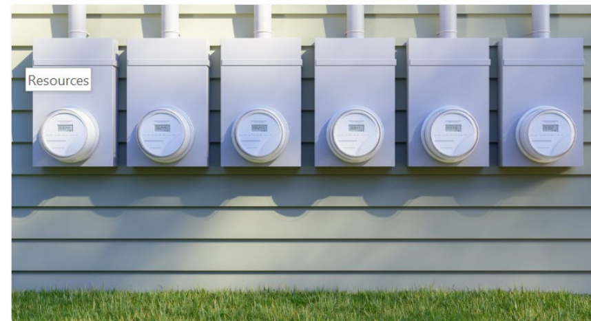
Front view of electric meters on building facade onurdongel via Getty Images
