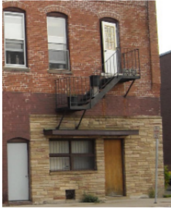
Fire escape and access accommodations should be placed on rear elevations if possible.
