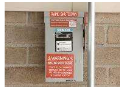
AC Disconnect/Rapid Shutdown
