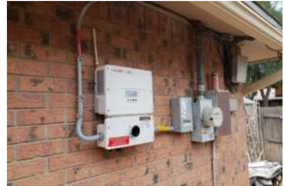
Photo from Green Solar Technologies
