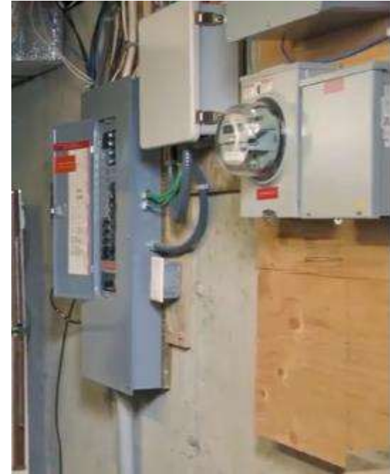
Main service panel board and meter. Photo from IREC
