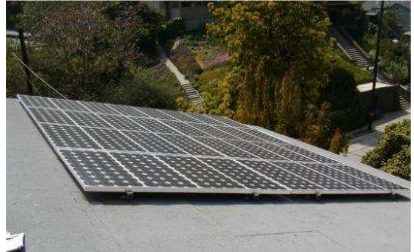
PV array. Photo from Brooks Engineering
