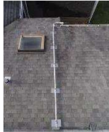
Conduits and Junction Box
